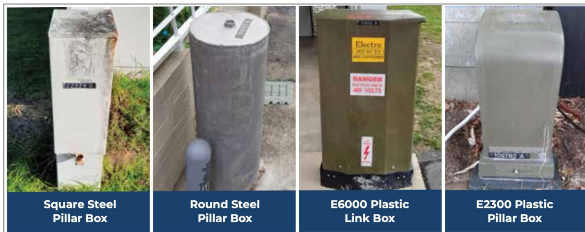
Figure 157: Example of pillar and link boxes
