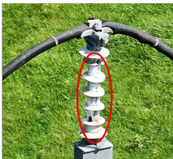
Figure 136: deterioration of 33kV polymer insulators
