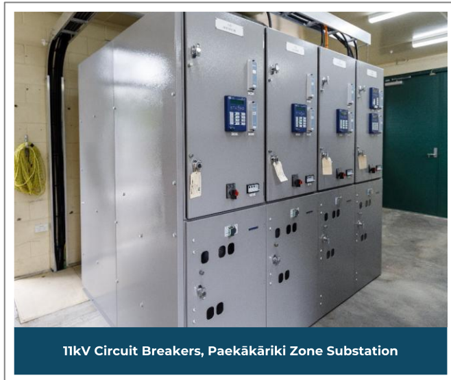
Figure 129: 11kV Indoor Circuit Breakers
