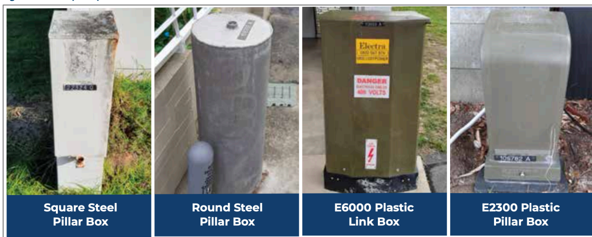
Figure 154: Example of pillar and link boxes
