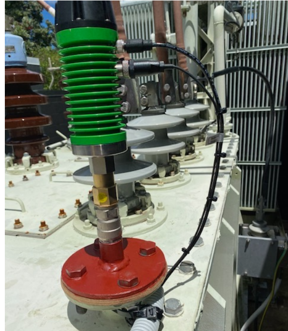
Moisture Probe Installed on a Power Transformer
