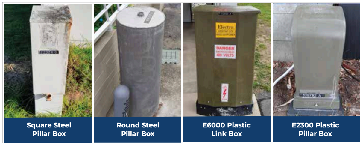
Figure 154: Example of pillar and link boxes
